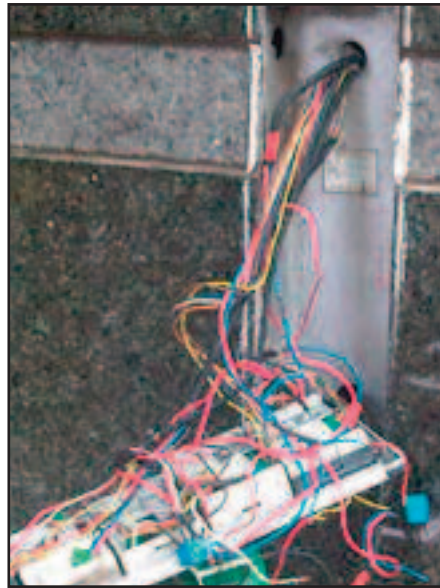
Not the way your building intercom should be looking like.
